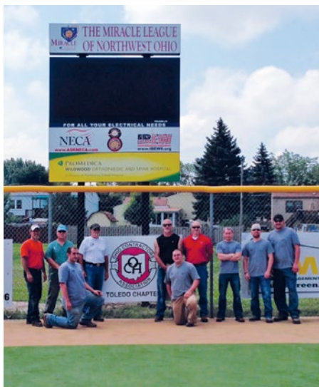
Local 8 members installed a new scoreboard and new electrical service at the Miracle League baseball fields.
